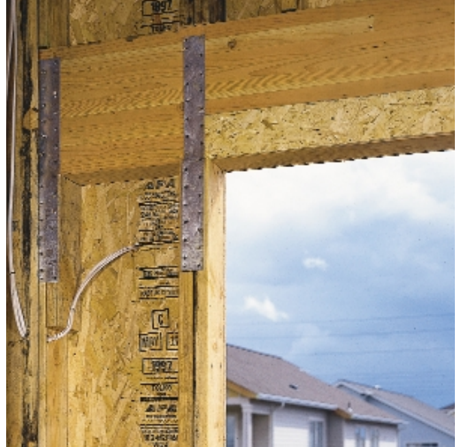
Glulam garage door header extends over adjacent narrow shear wall. (See Figure 4 for details.)
