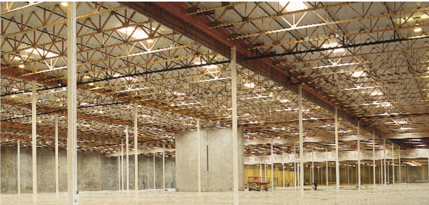
Panelized wood roof system featuring glulam beams and purlin trusses in the PepsiCo Distribution Center, Hayward, California.
