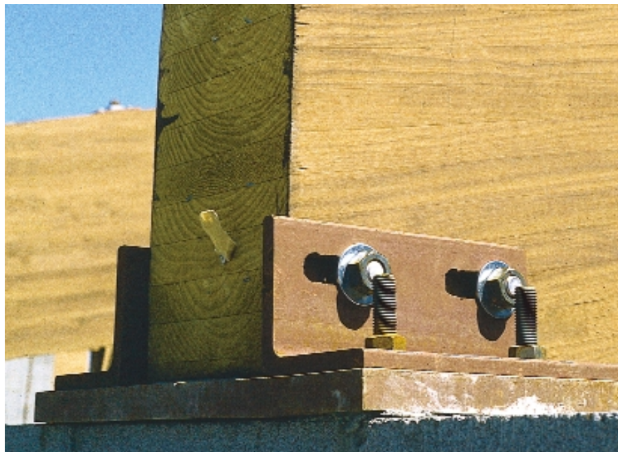
Slotted bolt holes permit horizontal movement of pitched and curved glulam beam.
