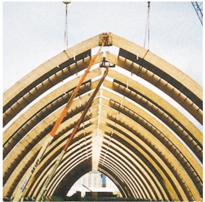
This 236,000-square-foot potash storage building in Portland, Oregon features APA EWS glulam arches.
