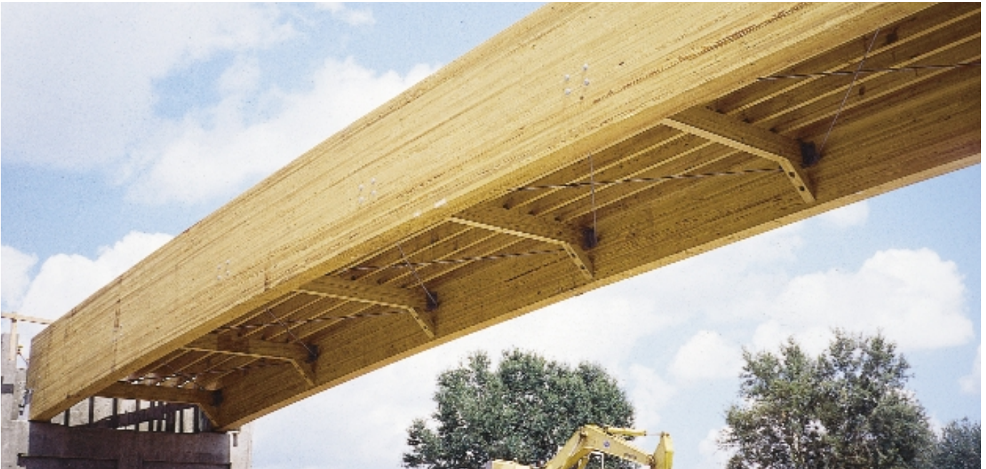
Glulam pedestrian and light vehicular golf course bridge under construction in Orlando, Florida.
