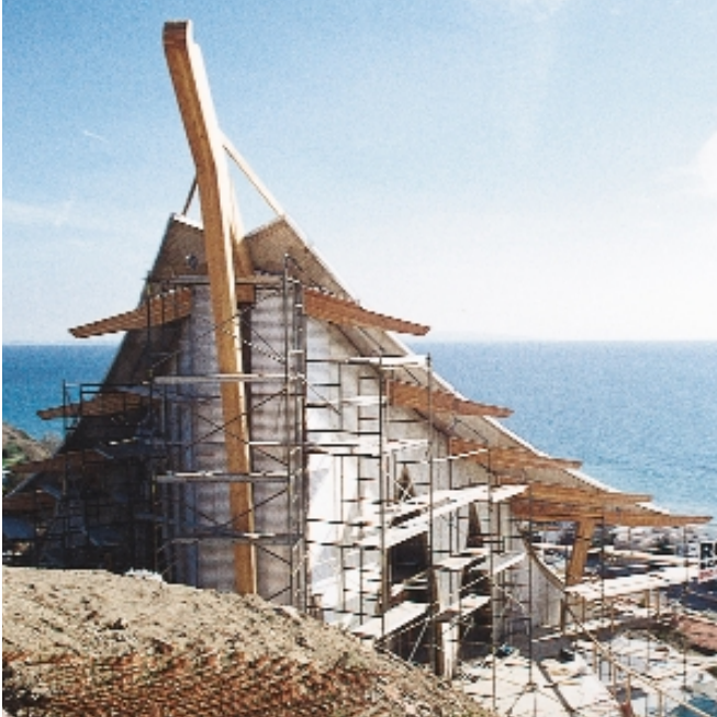
Long, curved custom glulam beams form the distinctive shape of this ocean view home in Malibu, California.
