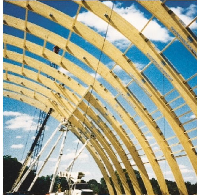
Glulam arches support the roof of the Chicago Bears practice facility in Lake Forest, Illinois.
